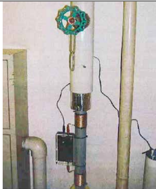
Vulcan 5000安装在工厂厨房
