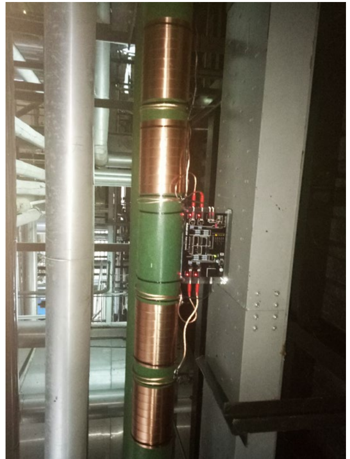
The Vulcan S25 was installed to treat the old chiller.
