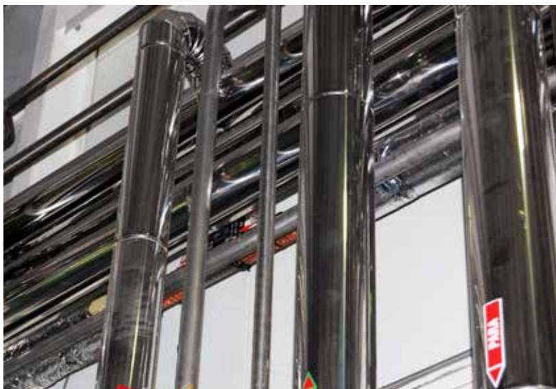
2 x Vulcan S25 were installed to treat the water for the whole brewery.
