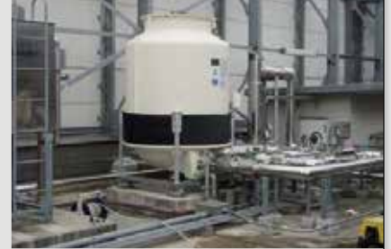
Cooling Tower C
