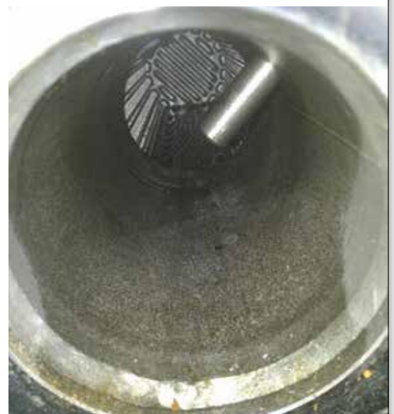
After 3 months – with Vulcan treatment. Up to now the installed pipeline needed no cleaning.
