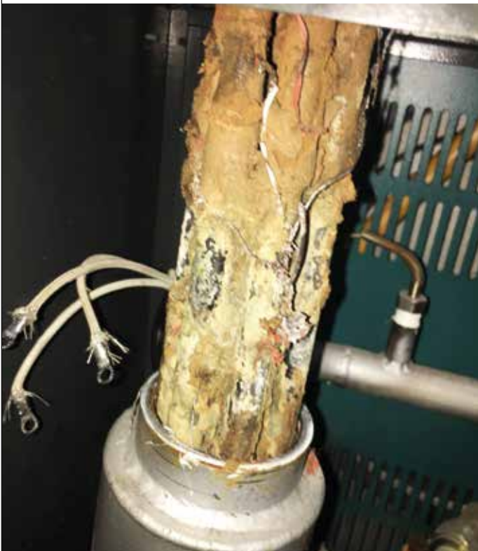
Untreated heat exchanger for 3 years.
