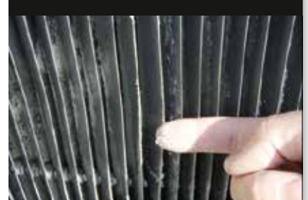
Silica could be removed by the high pressure water gun, and the remaining silica can be removed with a finger.
