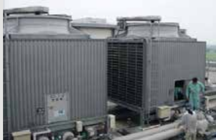
Cooling Tower A Cooling Tower B
