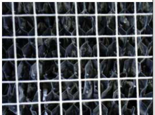
The photo above was taken of CT-1 about 6 weeks after the Vulcan was installed.
