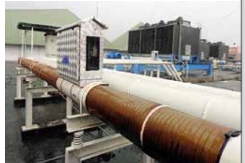
Vulcan S500 was located inside aluminum box and installed on a cooling tower main pipe.
