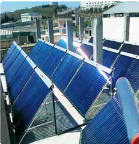
Solar heating panels of an apartment house
